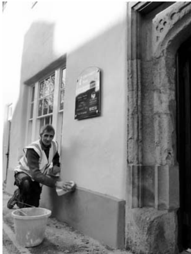
Foreman Roger Compton of building contractors A C Nurden Ltd, putting the finishing touches to external render
