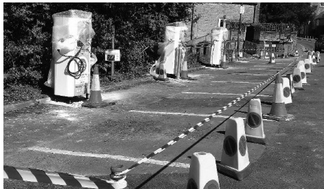
The new EV charging points being installed in the New Street Car park in mid April
