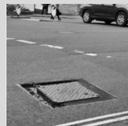
OCC – neck-breaking potholes, this one outside the Town Hall.
