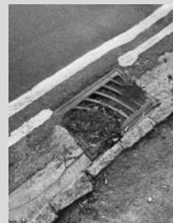
OCC – blocked drains and flooding surges down New Street (+London Road and more)
